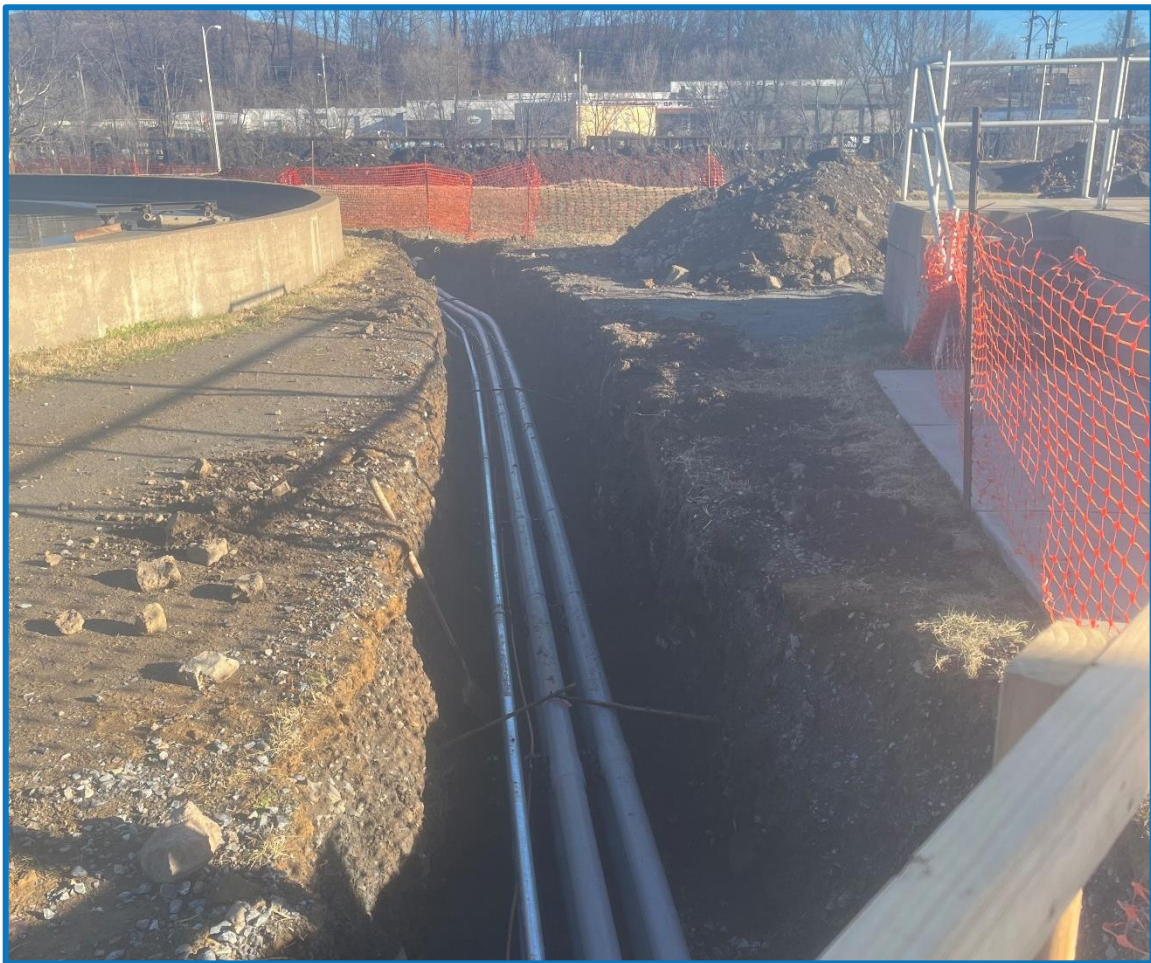
New Electrical Ductbanks between the Electrical Building and the Gas Purification Skid.
