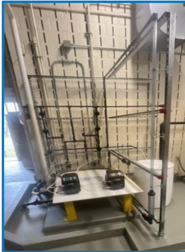
New Sodium Permanganate System – Front Street Pump Station
