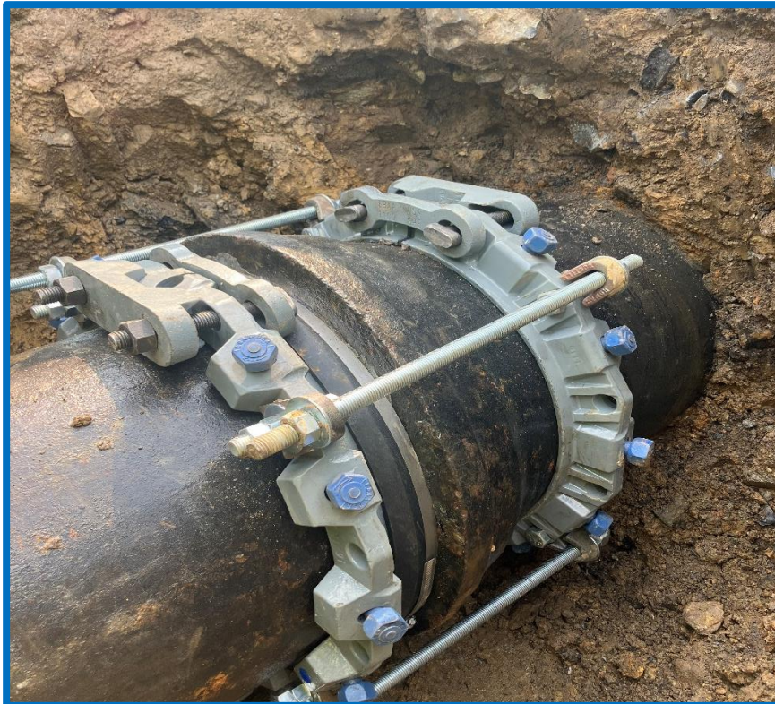
MJ 16-inch Bell Clamp at Capital
