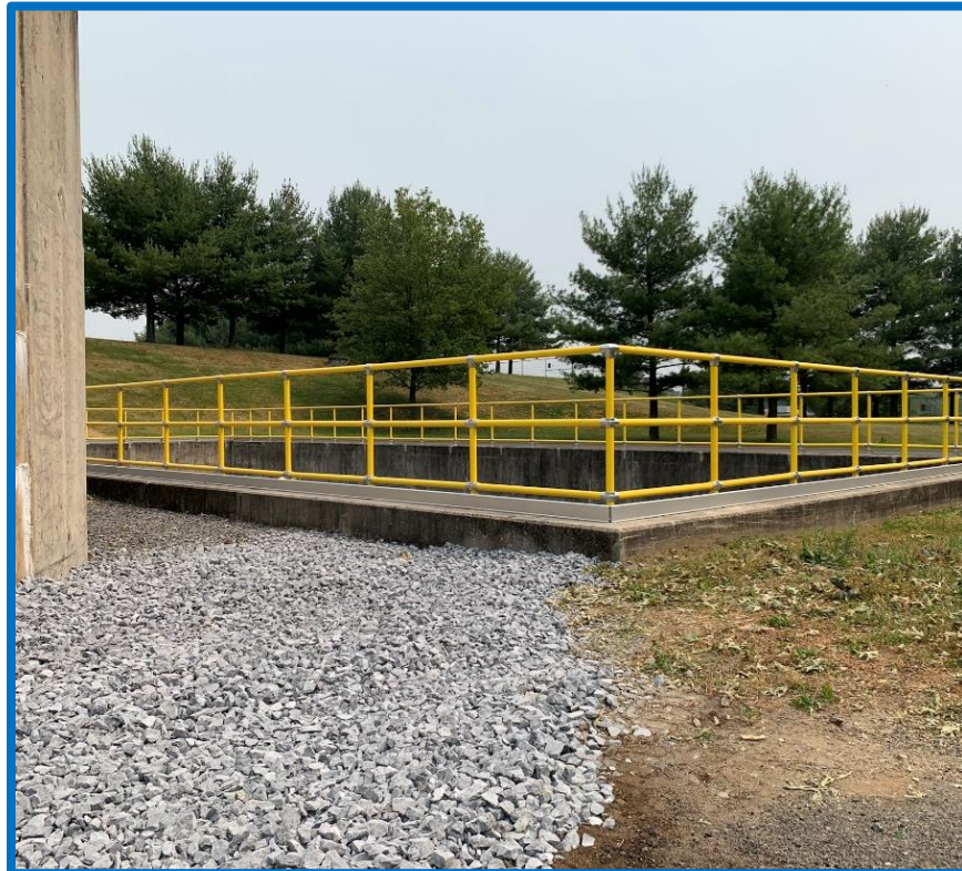
WSC New Backwash Pit Safety Speed-Rail® Railing System
