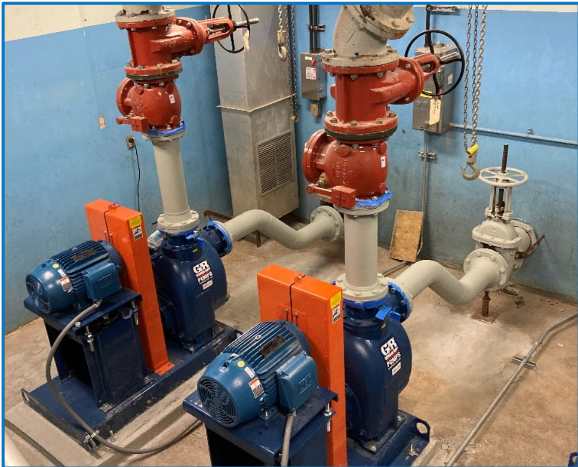
Newly Installed Pumps and Valves at the Plant Drain Pumping Station
