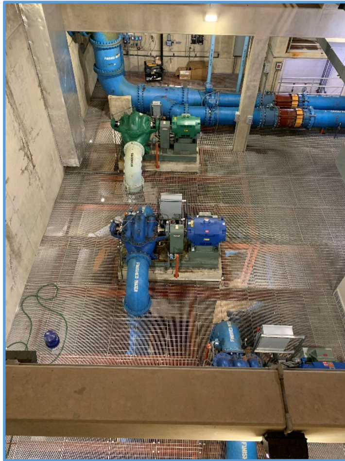
Finished and raw water pumps at WSC.
