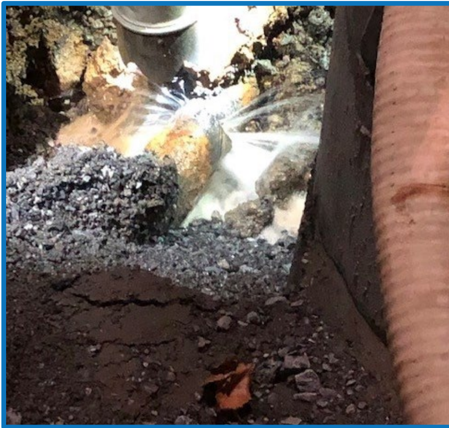
5 th and Seneca Streets – Water Main Break
