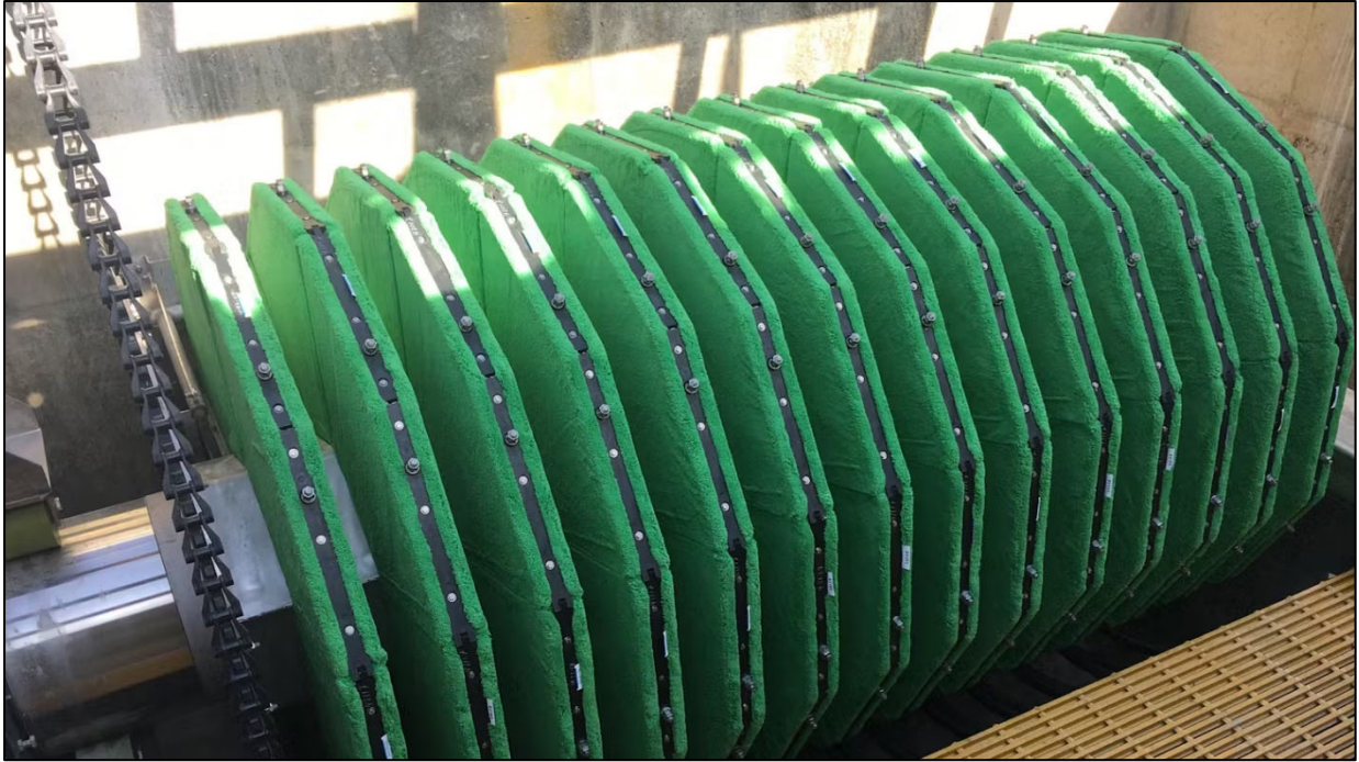
Figure 4.6-11: AquaStorm™ Cloth Media Filter by Aqua-Aerobic Systems
