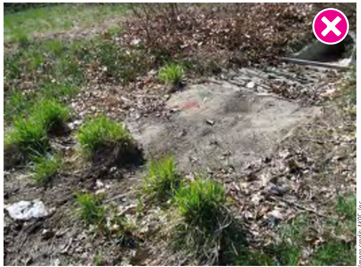
Eroded areas larger than 20 square feet in size, or settling more than 1 foot deep could be a potential indicator of significant problems.
