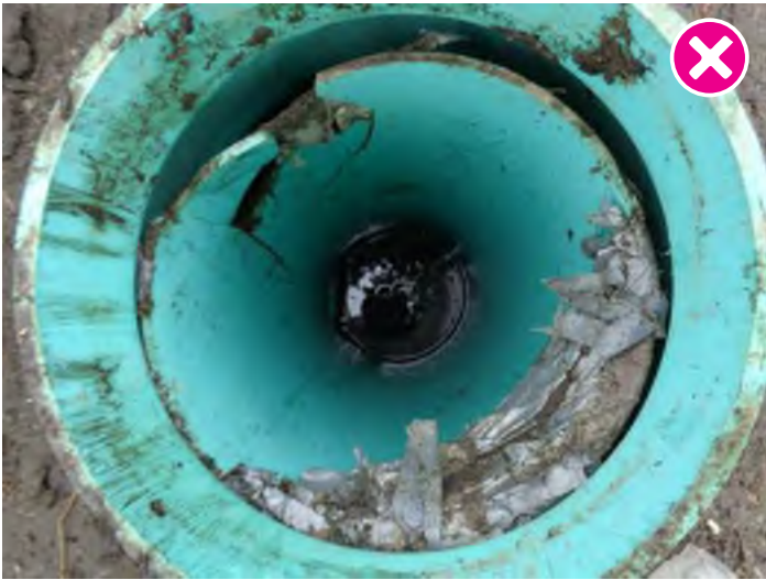
Pipes can be broken or damaged due to settling. Pipe repairs may require significant excavation and engineering.
