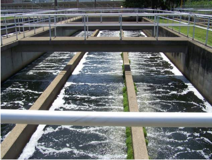
Figure 3.4-3 Photo of one Chlorine Contact Tank at the CRW AWTF
