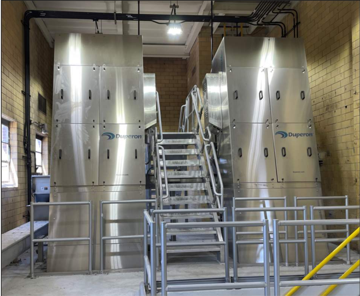
Figure 4.3-4 Front Street Pump Station Bar Screens
