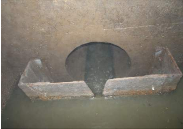
Regulating Chamber Effluent
