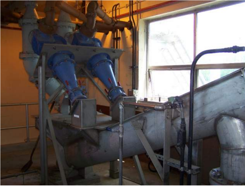
Figure 3.3-2 Photo of Classifier Unit at the CRW AWTF
